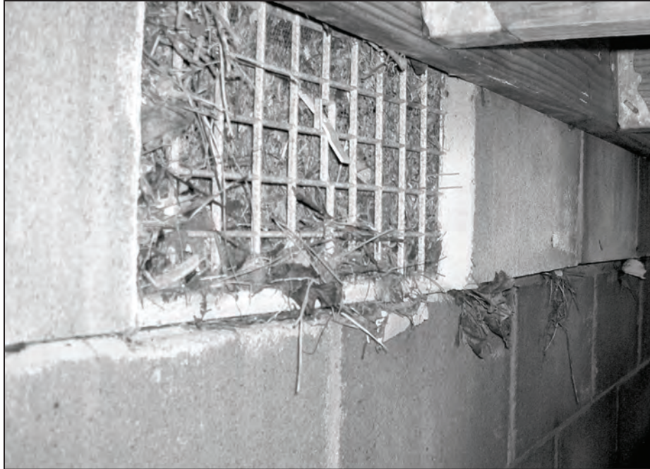
Figure 15. Typical air vent clogged by flood debris
